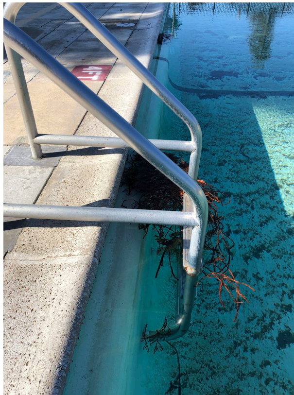
Ladder with More than 12 Inches of Clearance From Swimming Pool Wall
