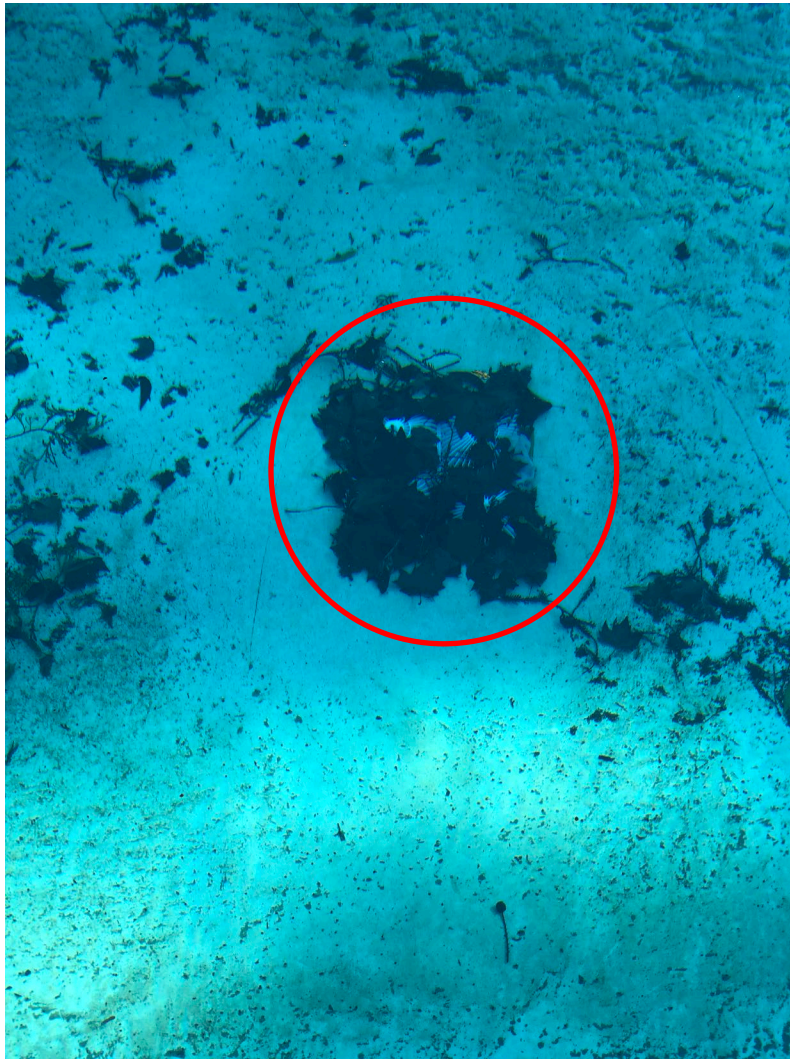
Main Drain for Swimming Pool
