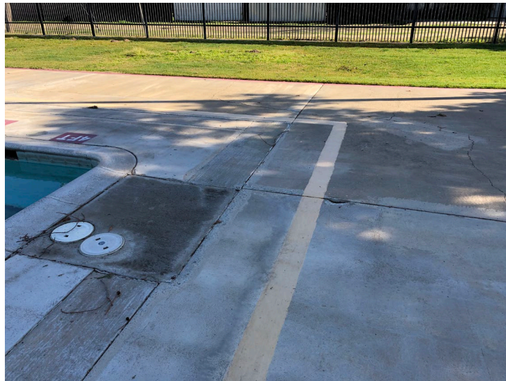
Swimming Pool Deck Has Visible Cracks and No In-Deck Drainage
