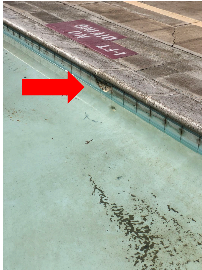
Chipped / Missing Swimming Pool Waterline Tile
