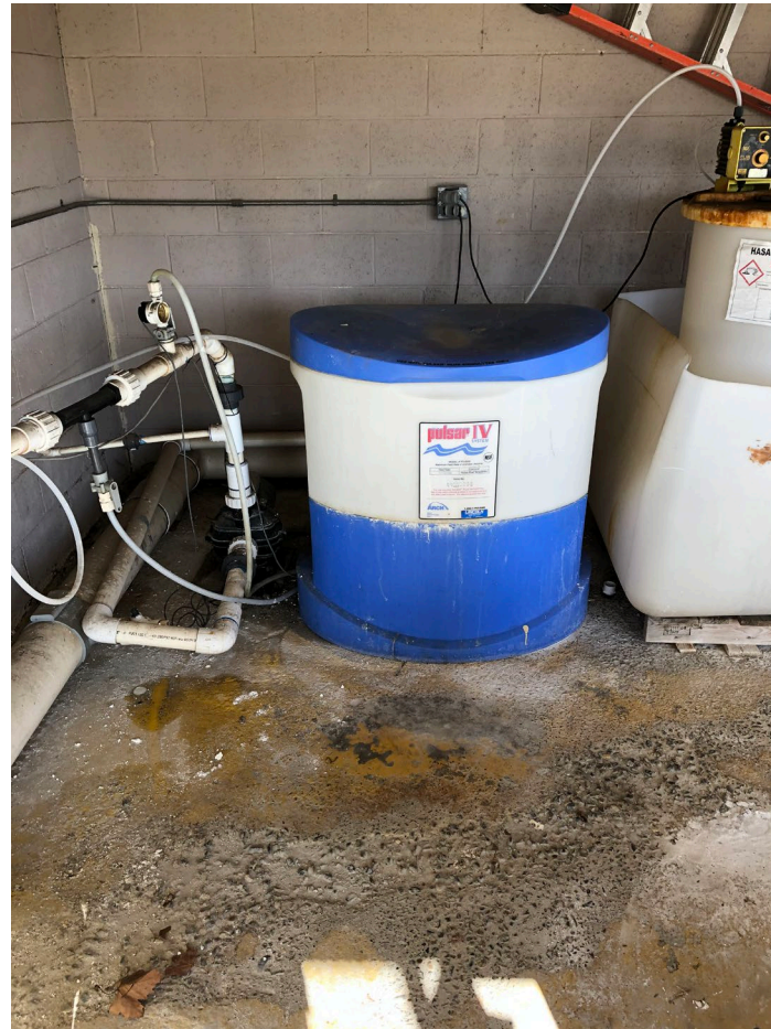
Chlorine System in Mechanical Enclosure
