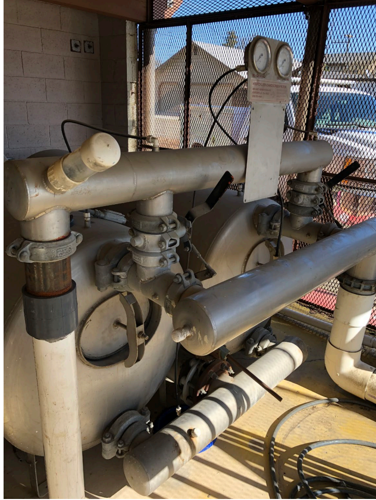
Swimming Pool Filter Tank System
