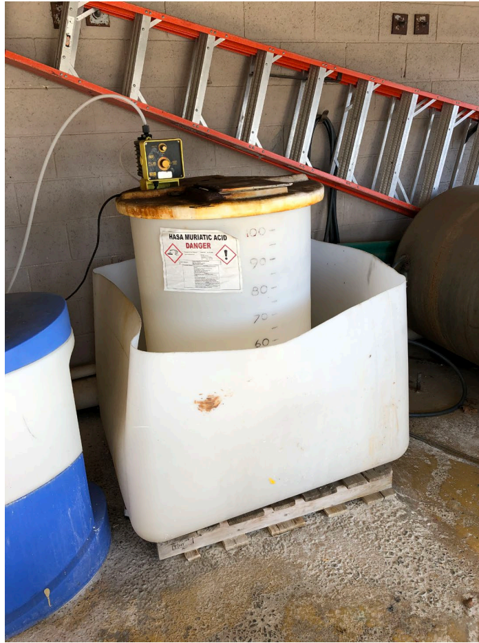
Acid System in Mechanical Enclosure
