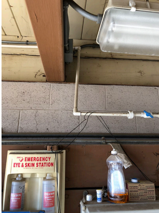
Emergency Eye Wash in Mechanical Enclosure
