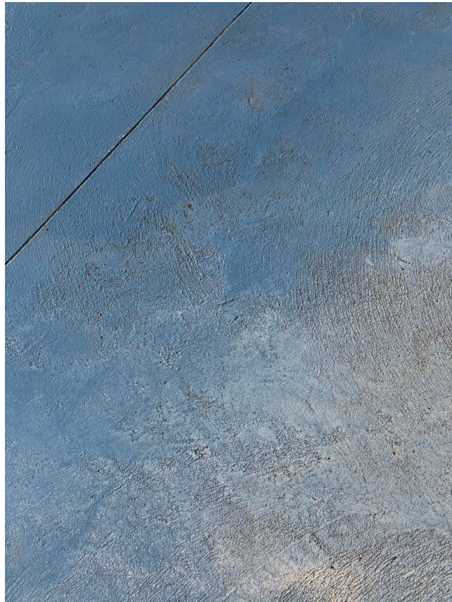
Existing Sprayground Surface
