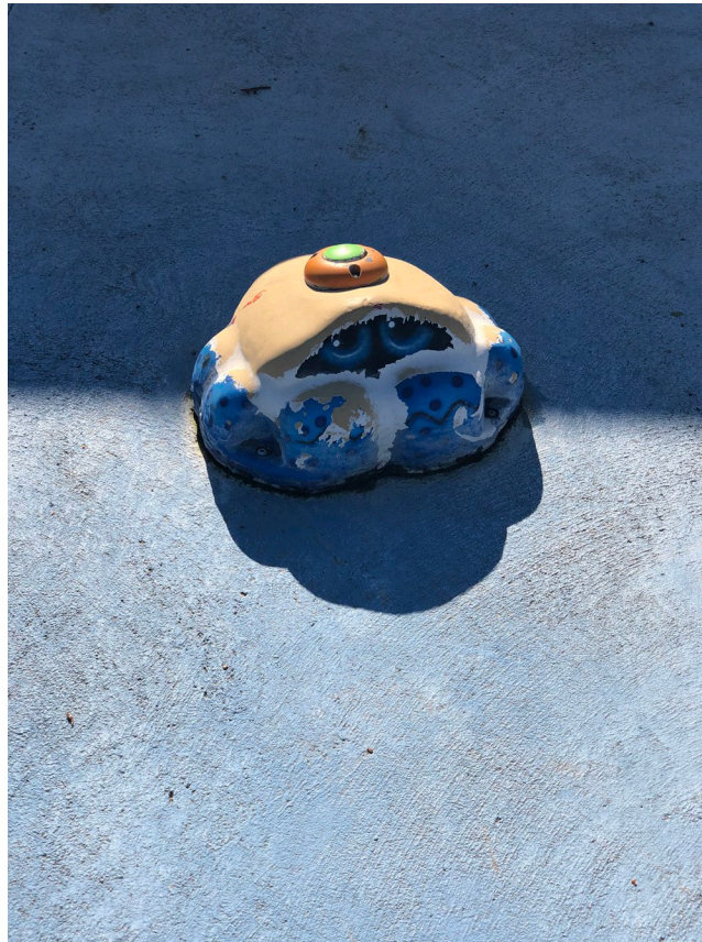
Faded Sprayground Feature
