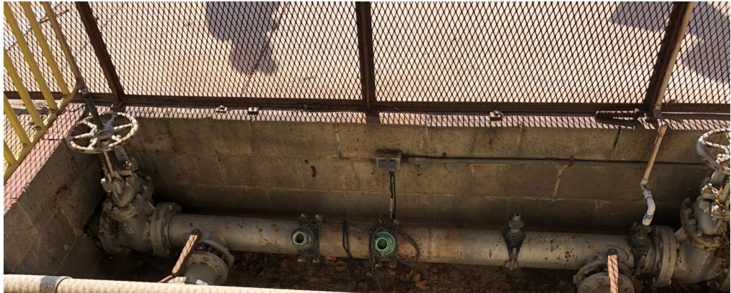
Steel Piping Corroding and Rusting
