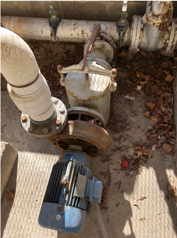
One of Two Swimming Pool Pumps, Motors, and Strainers
