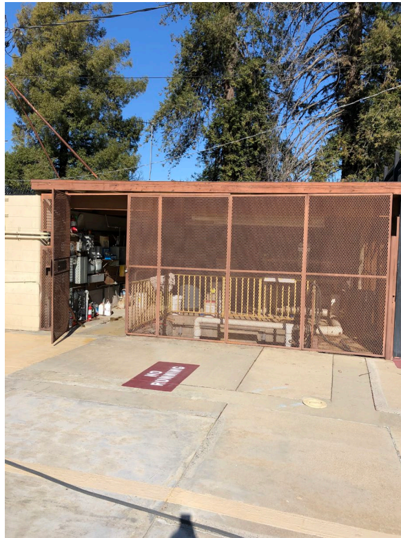
Swimming Pool Mechanical Enclosure
